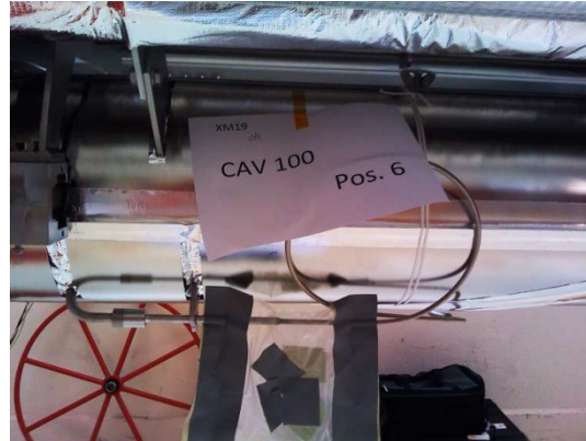
Leak on the 2K service tube of XM19 cryogenic distribution system
