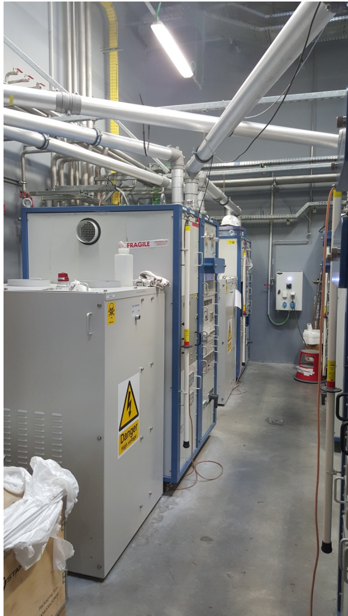
4 x 60 kW RF amplifiers
