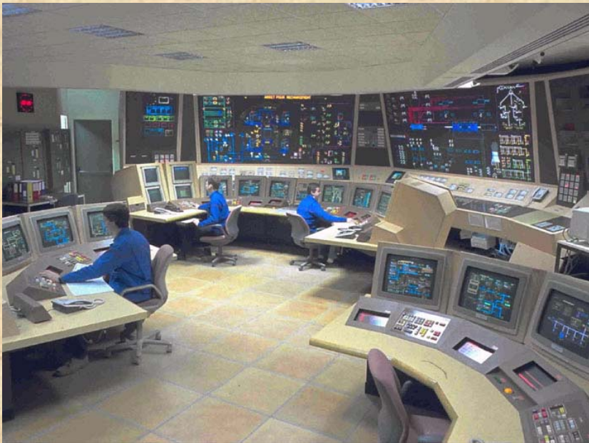
N4 Control Room
