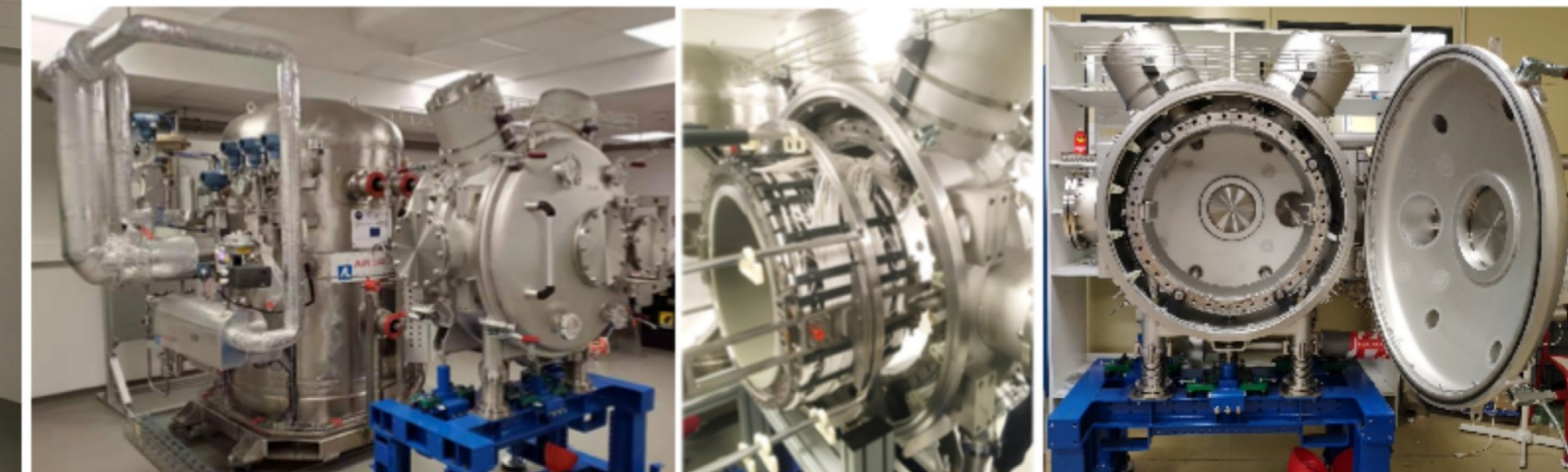
Installation @ Nantes CHU
