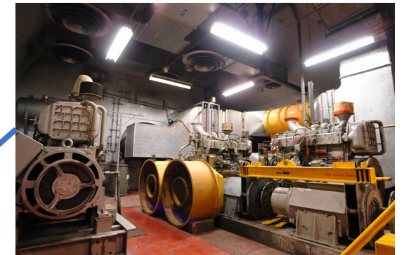
Generator room 500 m 2 , 7m height (-64m)
